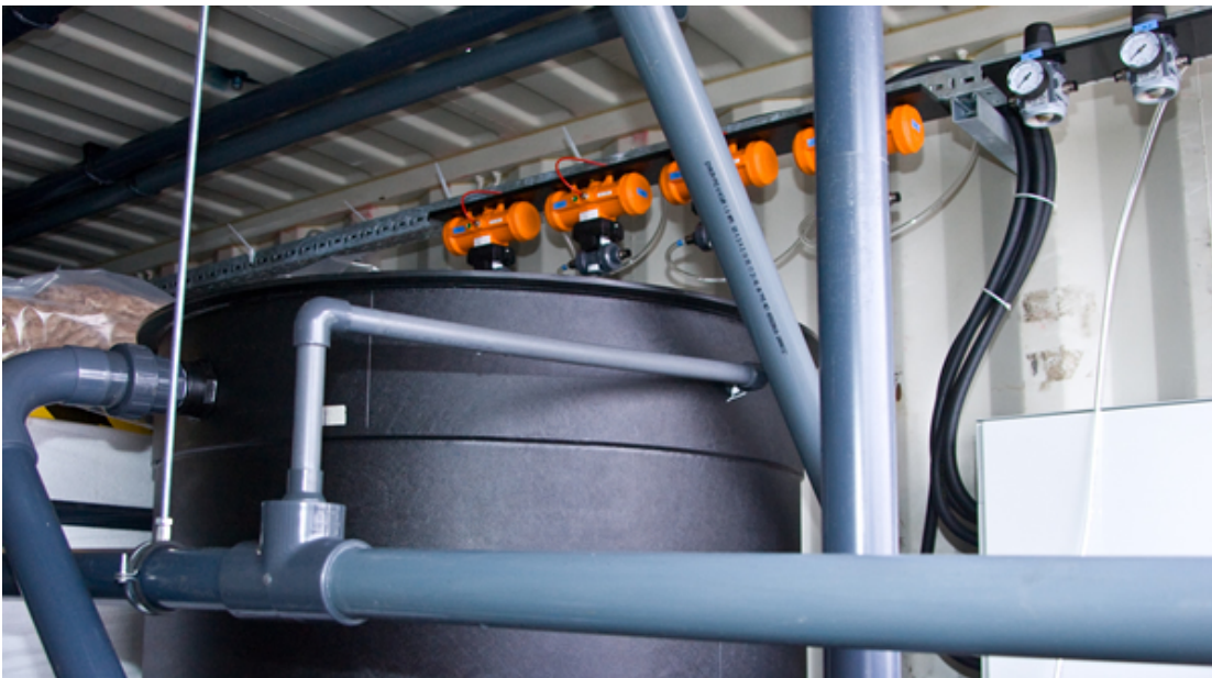
Prototype containerised core unit
